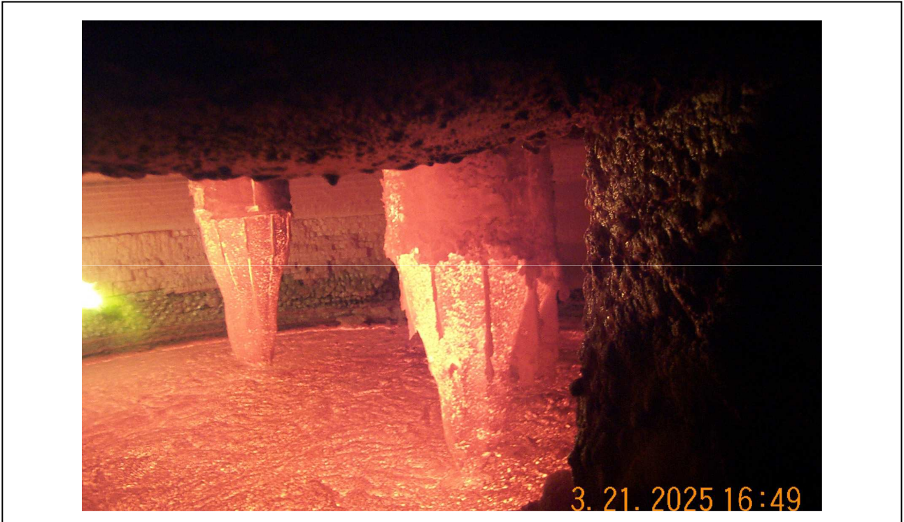
Figure 6: View inside slag cleaning furnace with bath level lowered
