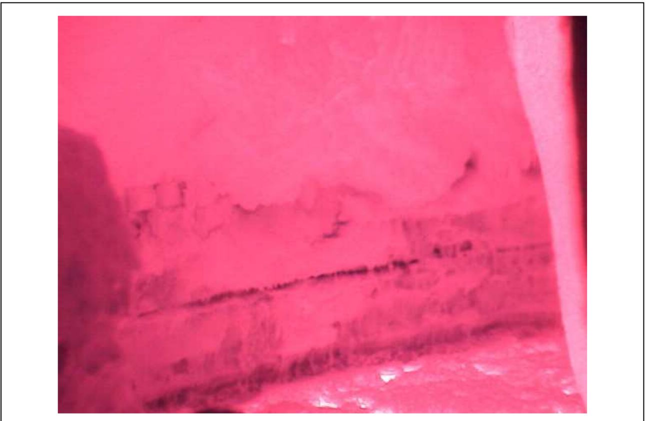
Figure 7: Close view of slag cleaning furnace sidewall showing freeze layer.
